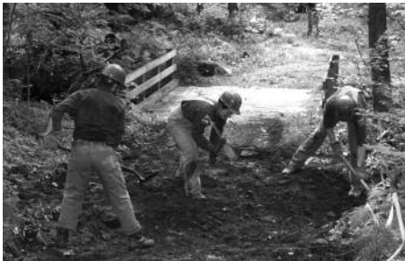
The VYCC crew installs a water bar on Burton Woods Road in Norwich.
