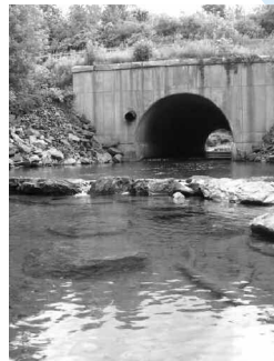
A rock weir below the Broad Brook culvert raises the water surface during low-flow conditions.
