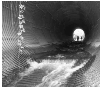
Wooden baffles in the Mill Brook culvert require routine maintenance.
